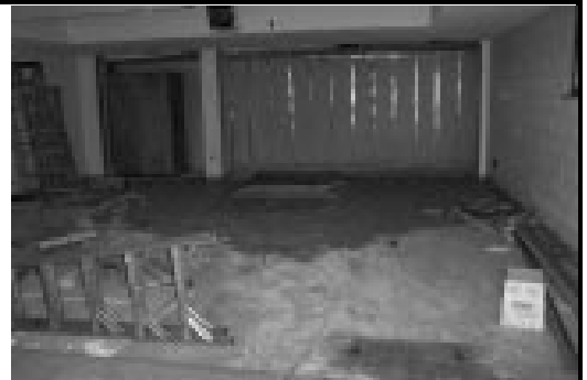
One of our first goals was to install a support system for underneath the new baptismal
